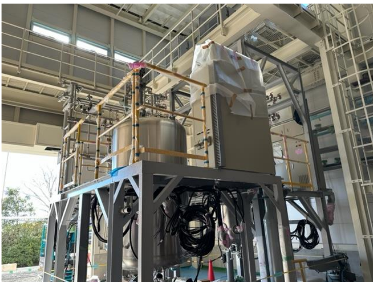
(Fig.3: Equipment installed in Bio-Foundry Research Center)
